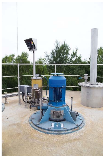
Stirrer digestion tower with central lubrication
