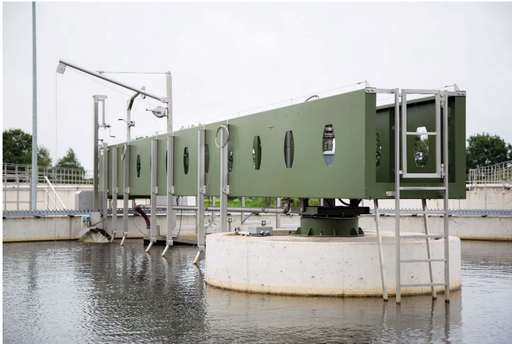
Secondary clarifier and round cleaner
